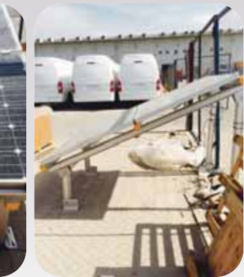
End user: Dubai Municipality Location: Dubai 5kwp, Solar off - grid system
