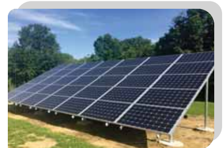
GROUND MOUNTED SYSTEM
