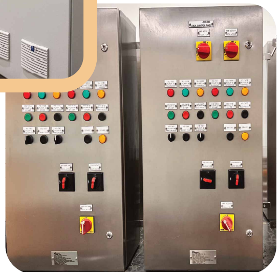
Local Control Panel
